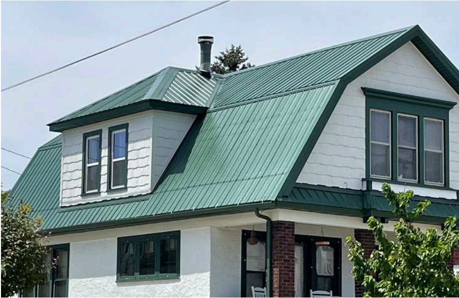
NOT RECOMMENDED corrugated or metal roofing, adding incompatible new chimney
