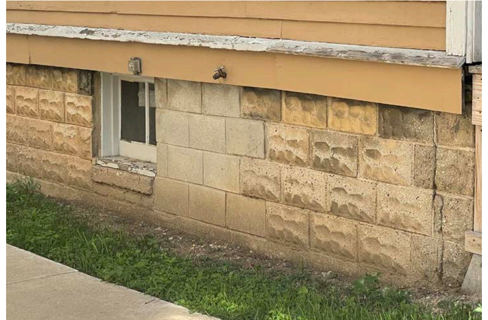
NOT RECOMMENDED masonry infill or repairs not matching the surrounding masonry
