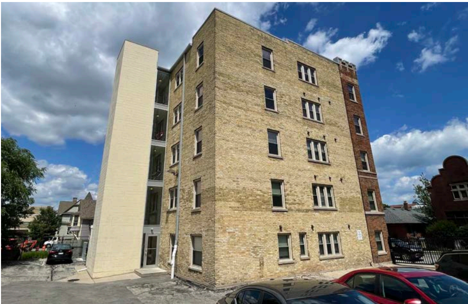
RECOMMENDED adding exterior stair or elevator tower to elevation not visible from street
