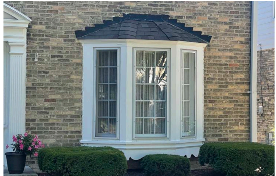
NOT RECOMMENDED replacing metal with substitute material that does not match
