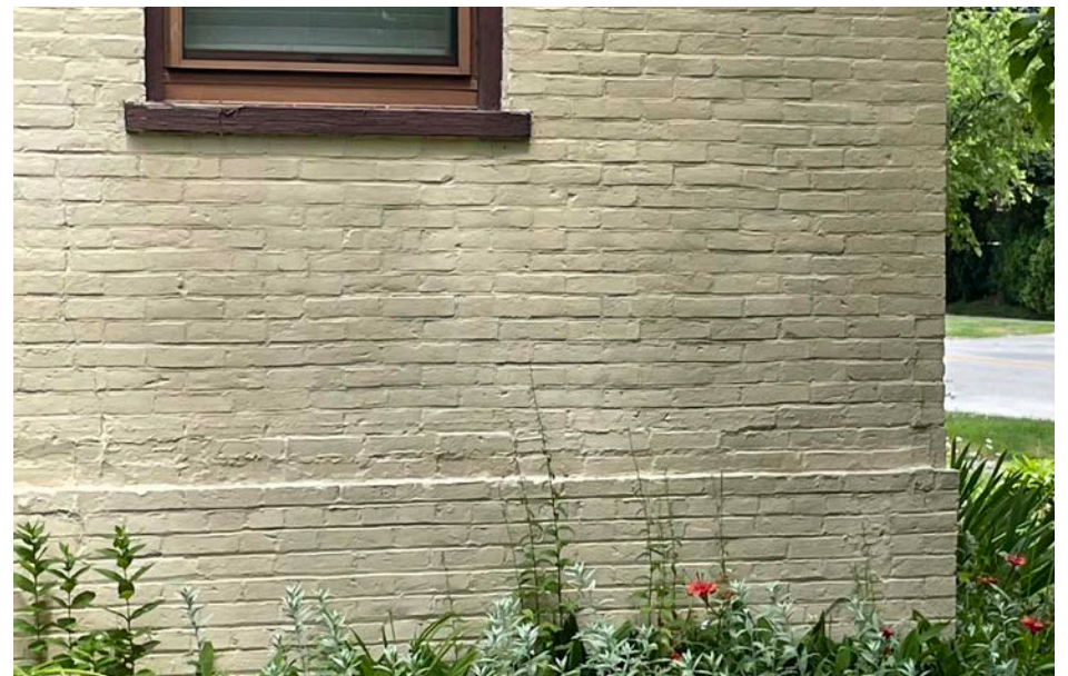
NOT RECOMMENDED applying paint to brick that has been historically unpainted
