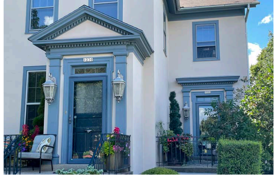
NOT RECOMMENDED New fixtures not compatible with scale of entrance
