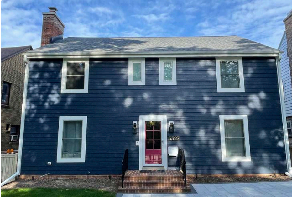
NOT RECOMMENDED replacing with incompatible substitute materials
