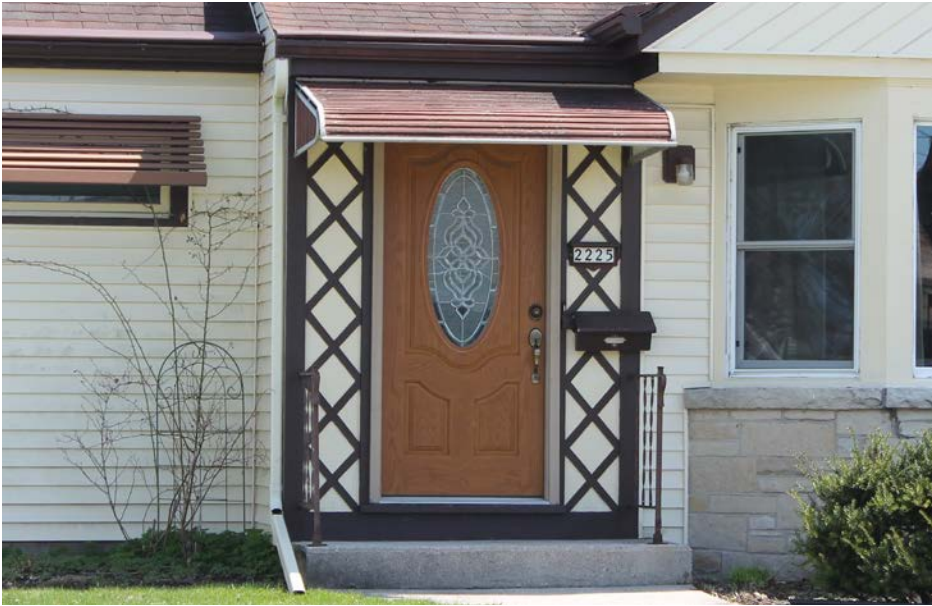
NOT RECOMMENDED incompatible replacement door
