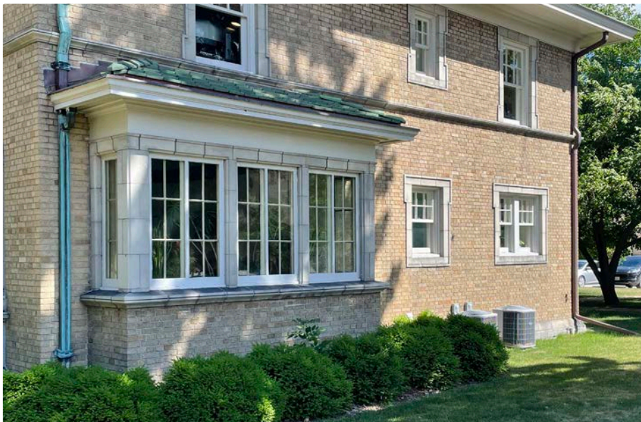
RECOMMENDED placing air conditioning compressors not visible from the street
