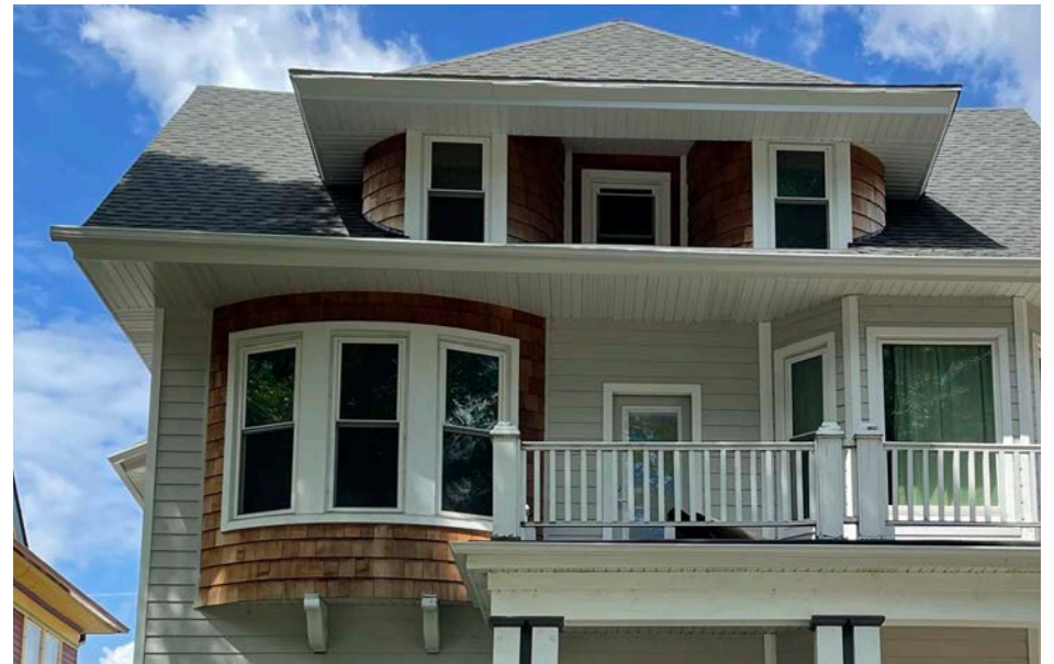
NOT RECOMMENDED unpainted wood finishes that were historically painted
