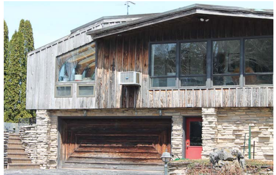
NOT RECOMMENDED mechanical units visible from the street
