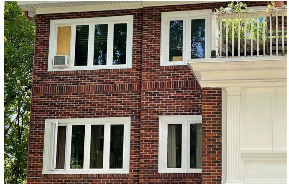
NOT RECOMMENDED vinyl windows in incompatible style for house
