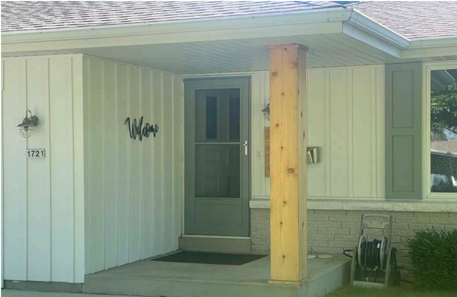
NOT RECOMMENDED covering wrought iron porch post with wood
