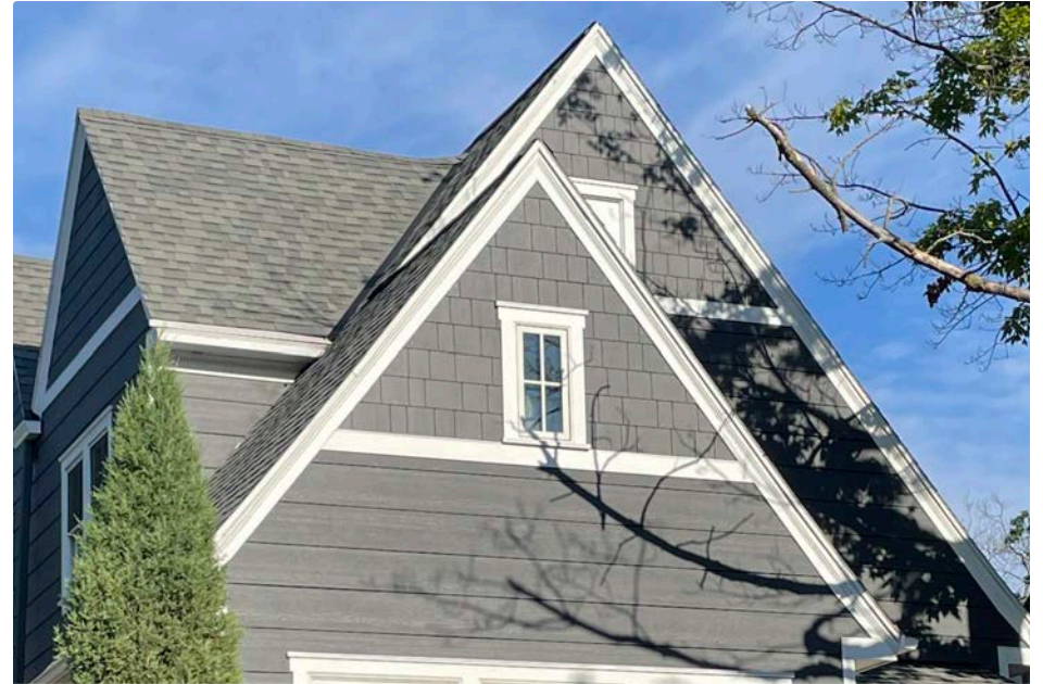
NOT RECOMMENDED replacement siding with faux wood grain texture
