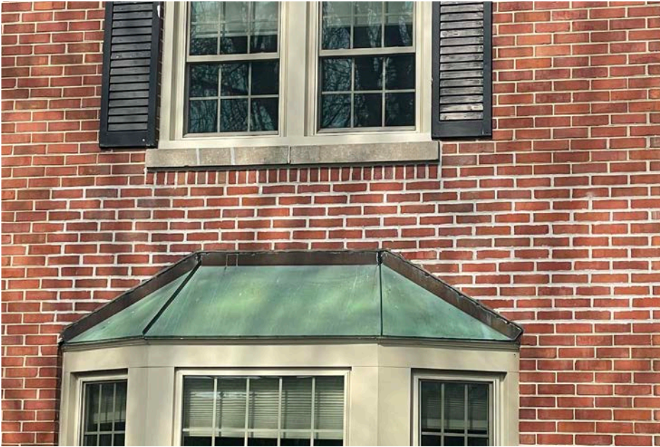
NOT RECOMMENDED not matching new mortar color, texture, profile & width of the old
