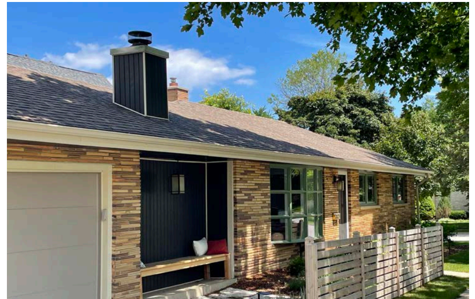
NOT RECOMMENDED adding highly visible new features (chimney) to roof
